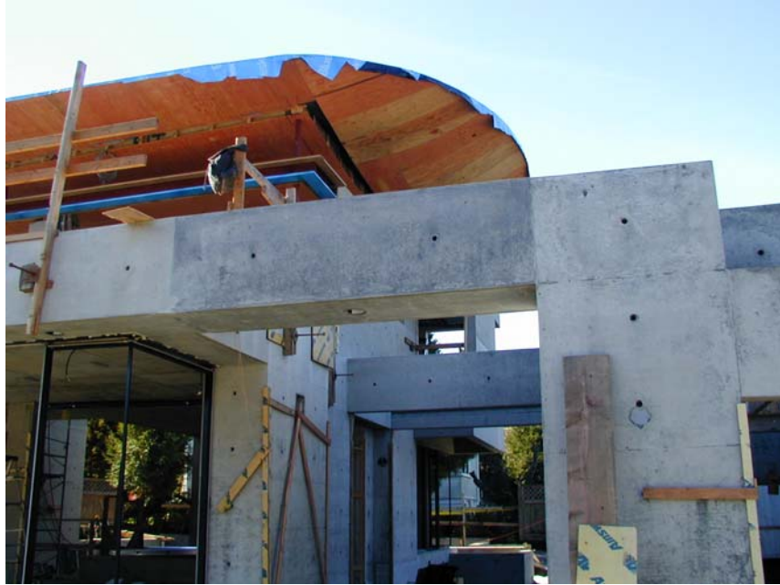
Figure 4: Discolored HVFA Concrete Panel Poured during Cold Weather Period
