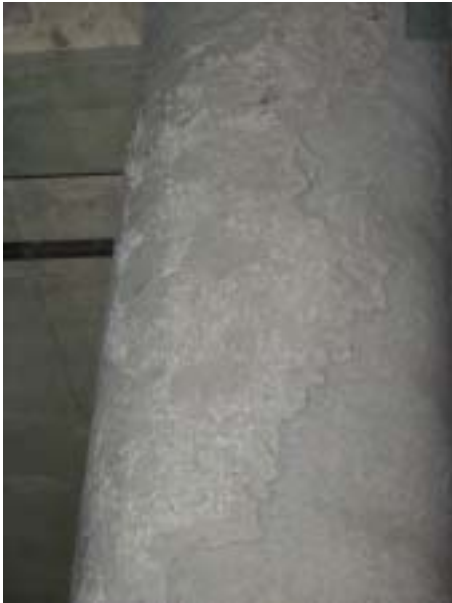
FIGURE F4.8 HONEYCOMBED COLUMN
