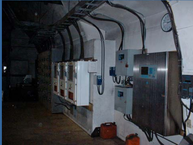
Fully Automated Control System
