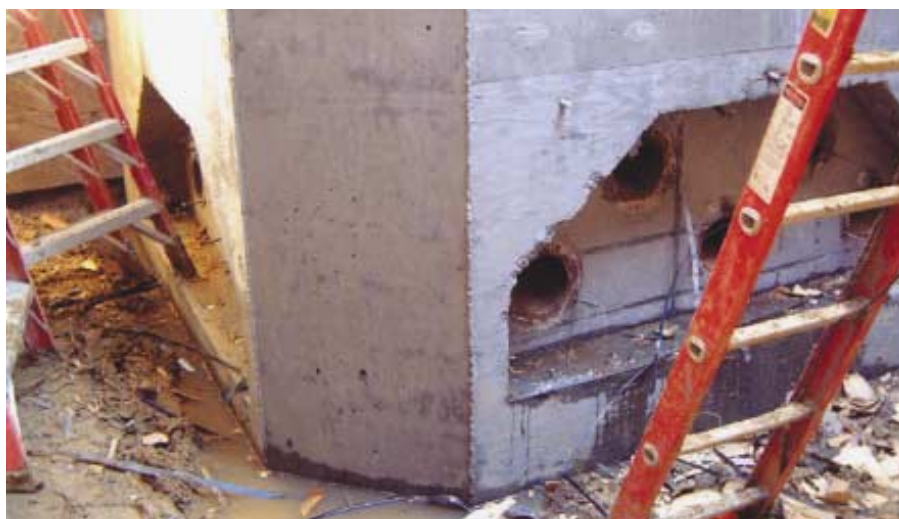
Fig. 5: Close-up of corner foundation with post-tensioning ducts. Notice the smooth finish on the exterior surface
